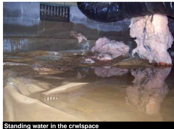
Standing water in the crawl space
