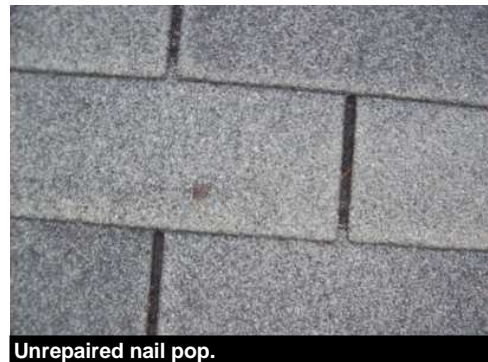
Unrepaired nail pop.
