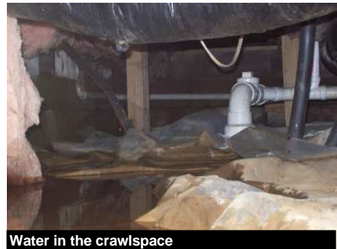
Water in the crawlspace
