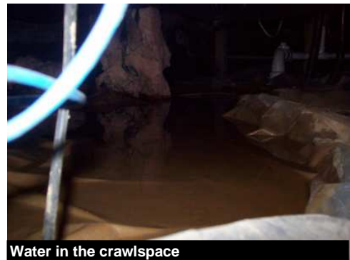
Water in the crawlspace
