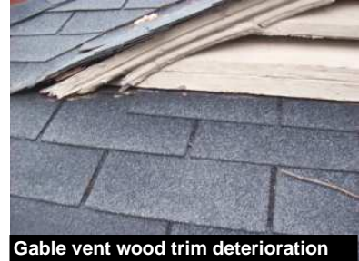
Gable vent wood trim deterioration
