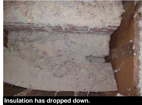
Insulation has dropped down.
