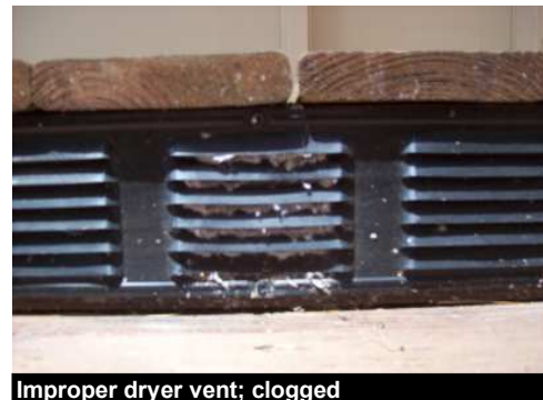
Improper dryer vent; clogged
