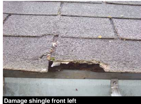
Damage shingle front left
